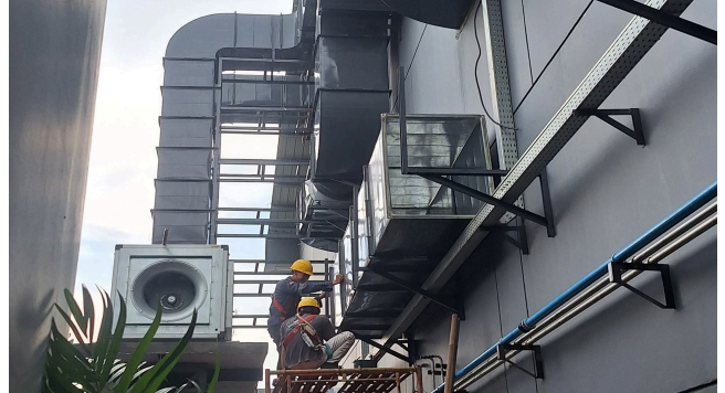
Ducting Supply, Installation & Maintenance
