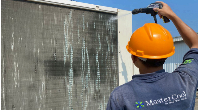
HVAC Supply, Installation, Troubleshooting & Maintenance
